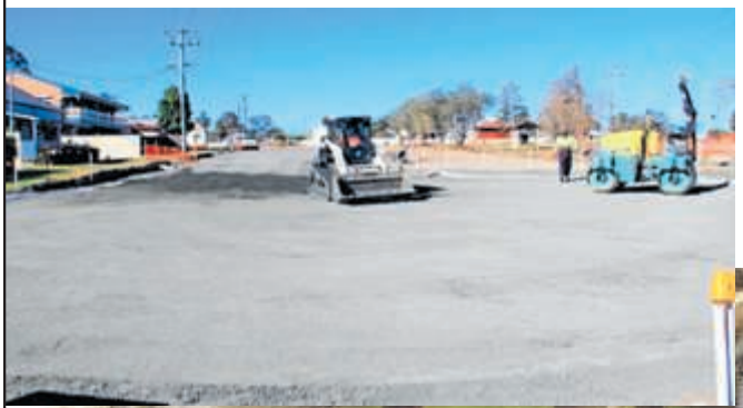
Drainage infrastructure & the road re-alignment will help parking & traffic movements. The work is being funded by 'Roads to Recovery'
