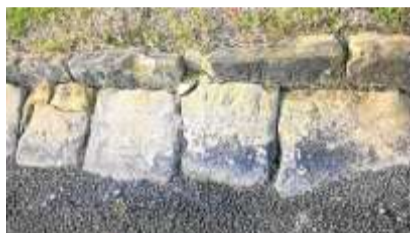
• Sandstone guttering lifting in Branxton
