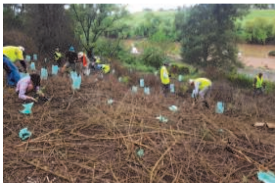
■ Photos above: Top photo - the volunteers after a hard days work. Middle photo - before & above after.
